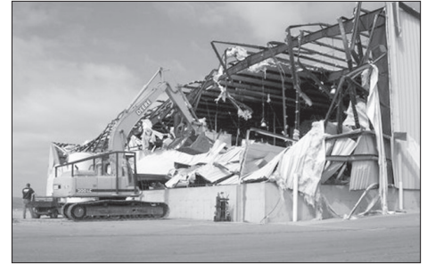
Co-Line's middle building had steel siding from the roof and south side ripped off.
