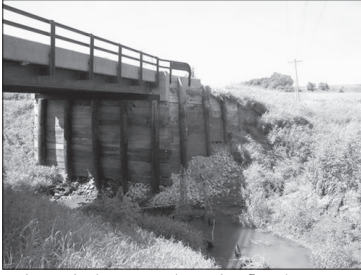
A huge hole, carved out by flood water, forced the county to temporarily close this bridge on Cordova Ave.
