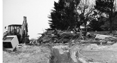
Top to Bottom: Shed demolition, the house before tear-down, half the house is gone, finally only a pile of rubble is left next to the old stumps.
